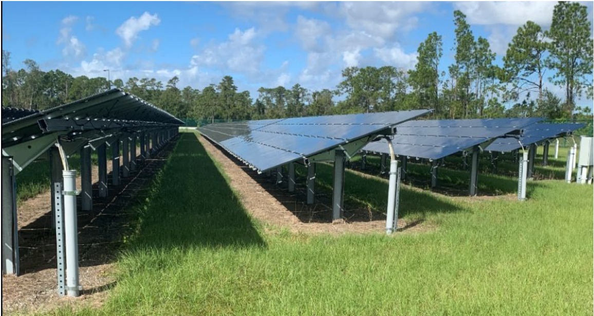
Figure 1: Duke Energy Solar Farm
